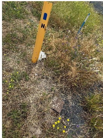
Figure 6 – Ex hydrant (east most hydrant on William St)
