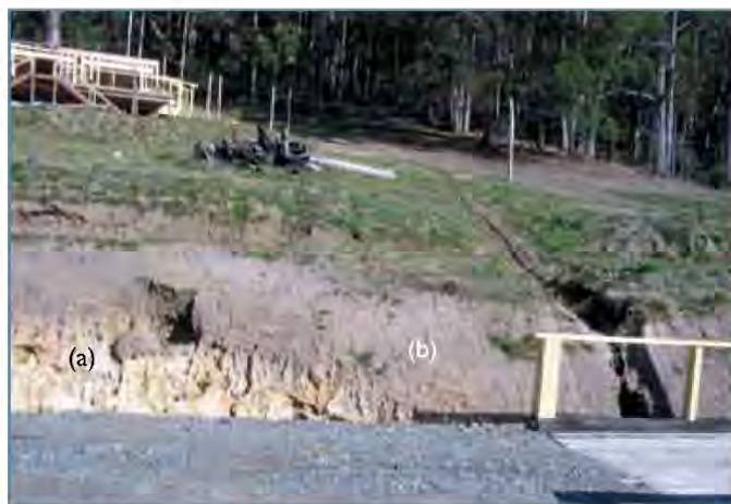
Figure 13. The severity (or sodium content) and depth of dispersive subsoils can vary considerably over short distances. (a). At this site highly dispersive subsoils exist meters away from (b) non-dispersive soils.
