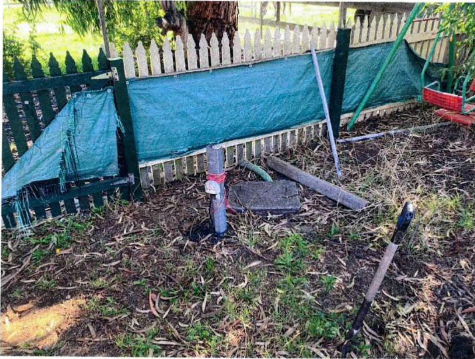
Plate 2 – greywater sump tank - fitted with a submersible pump.
