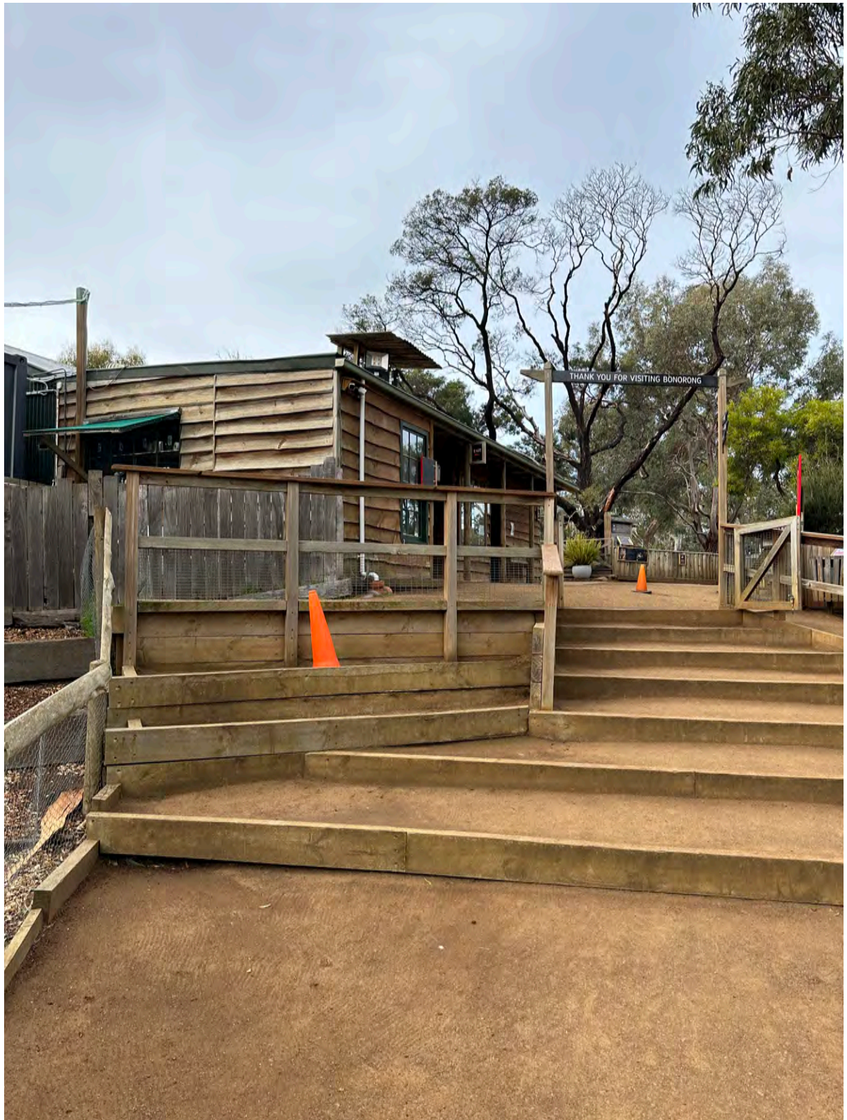
Fig 20. The new ramps will allow wheelchair access and walking frames and prams. The ramp will move across the undulating terrain.
