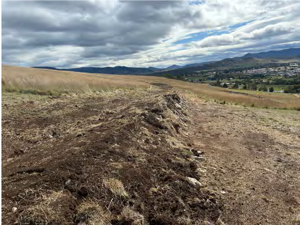
Fig 34. New landscaping swales to aid in hydrology and a new tree planting program to encourage wildlife and redevelop wildlife corridors between the Jordon River and the Meehan Range.
