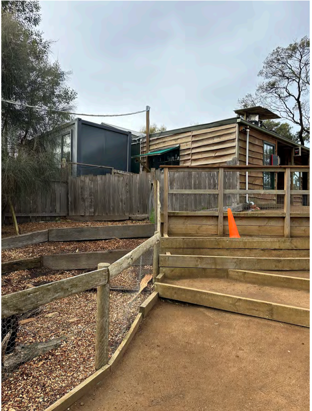
Fig 21. The new ramps will allow wheelchair access and walking frames and prams. The ramp will aid in moving across the undulating terrain.
