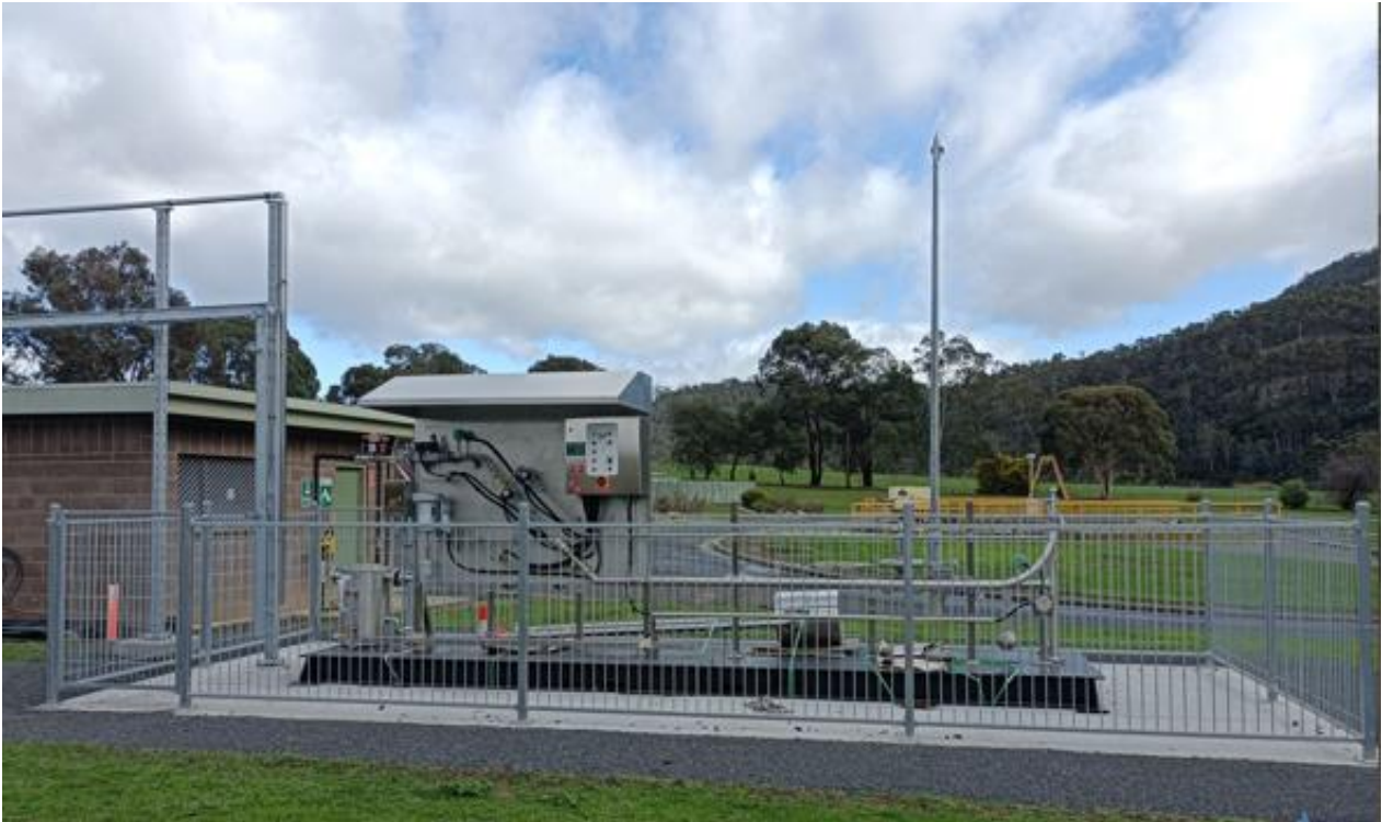
Figure 3: an image of the biogas flare to be installed at Green Point STP.
