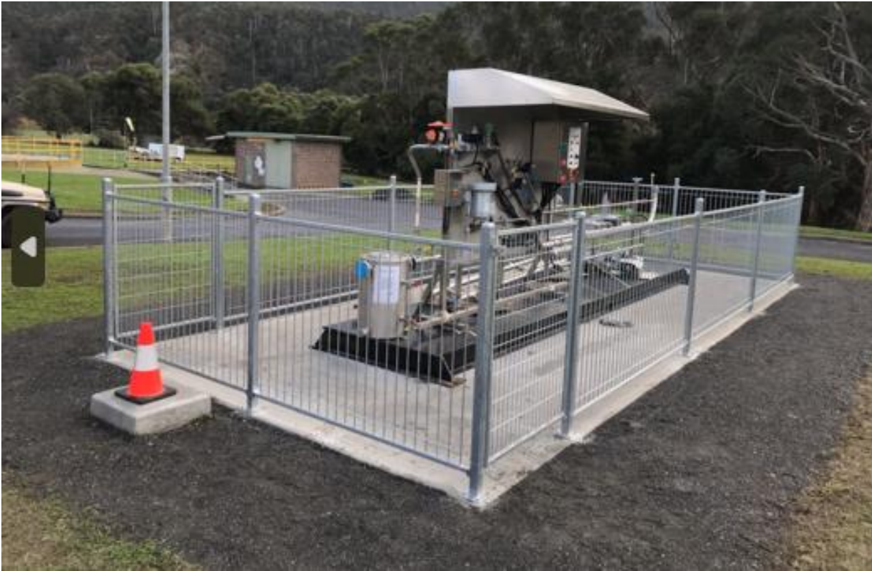
Figure 2: an image of the biogas flare to be installed at Green Point STP.
