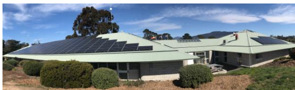
15kW addition to Council Offices in 2021 brings total generation capacity to 65kW, October 2021
