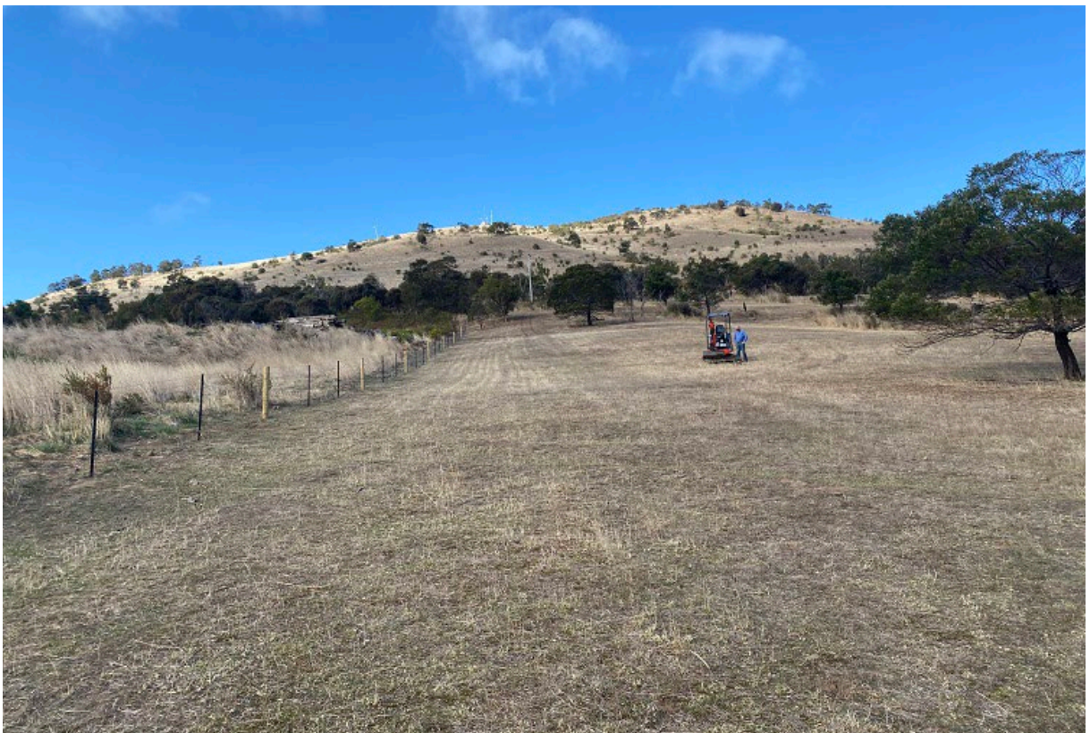
Plate 4 (below). View on proposed Lot 2 upslope to the south from near the lower property boundary. The excavator is digging test pit B.
